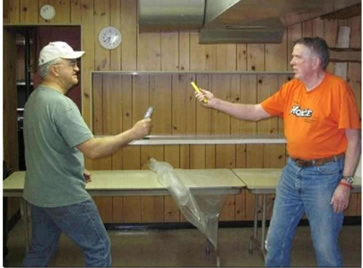
Pat and Bert sparring during the downstairs ceiling project at the church
